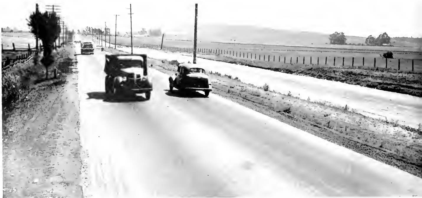
View of new four-lane highway between Napa Wye and Vallejo before paving operations. New lane is on right
